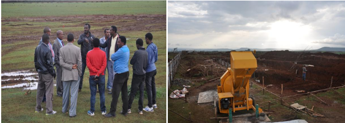
DMU top management delegate led by Dr. Tilaye Gete making supervision in Health campus construction site.
